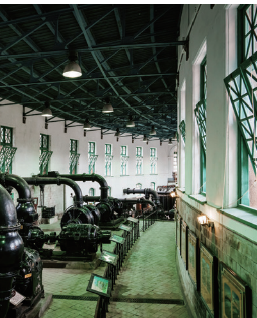
Pumping station machinery
